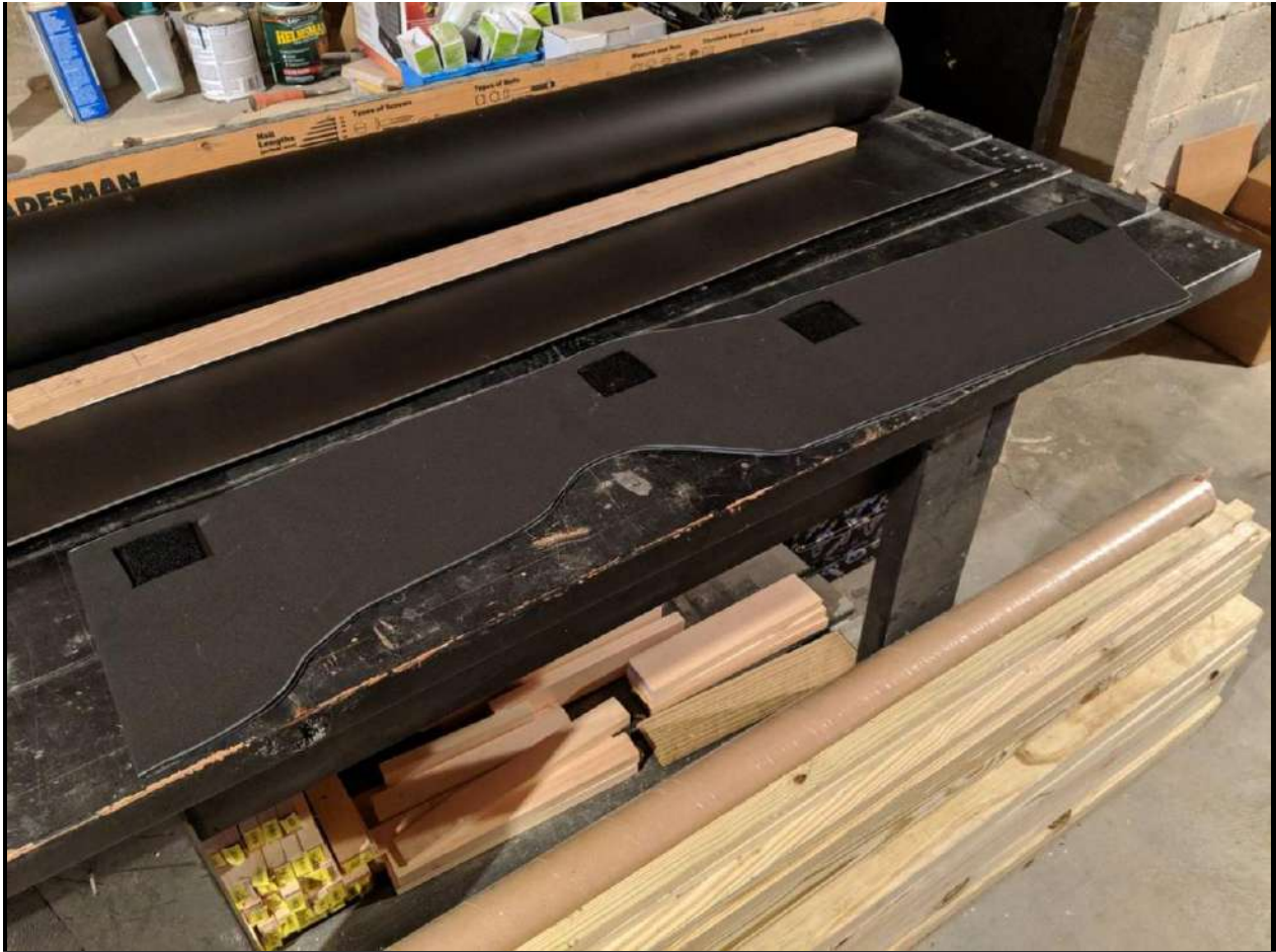
Here, the CCF, with the holes cut for the velcro tape, is laid onto the MLV for the passenger's side of the center tunnel
