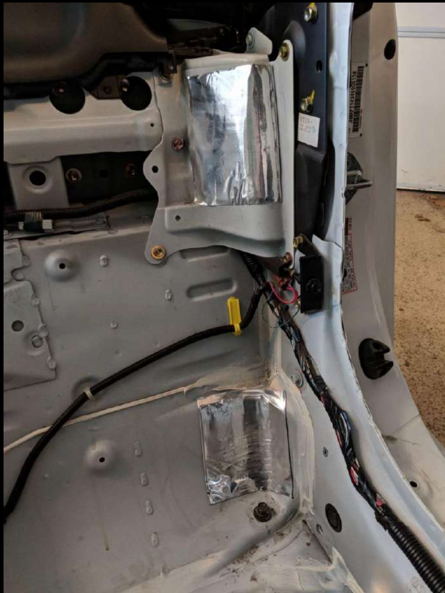
CDL tiles were applied to the interior driver's side quarter panel itself
